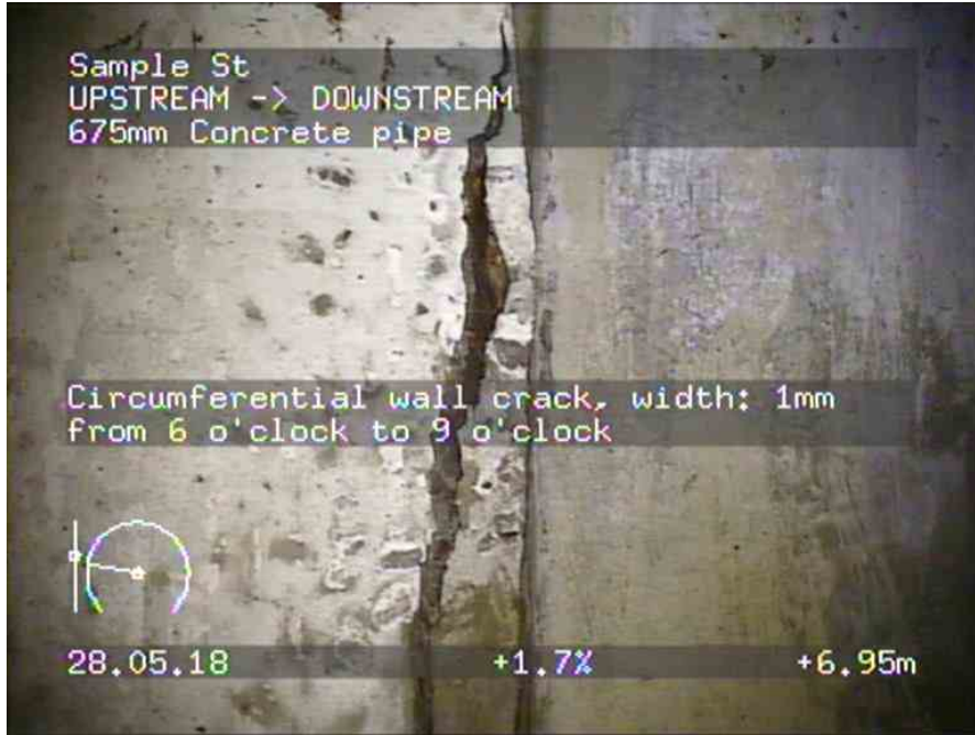
LINE 1_bebc146b-f2ef-45e3-b51c-7c5bde17b2b1_20180528_163535_506.jpg, 00:03:12, 6.95 Circumferential wall crack, width: 1mm from 6 o'clock to 9 o'clock
