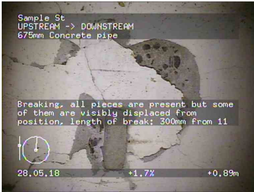
LINE 1_85427e28-b870-4ad3-9bcc-0ccd0441c95c_20180528_163226_386.jpg, 00:00:51, 0.89 Breaking, all pieces are present but some of them are visibly displaced from position, length of break: 300mm from 11 o'clock to 1 o'clock
