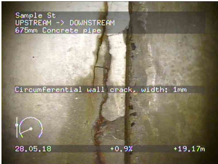
LINE 1_c92a64c4-728d-4ddf-aad3-a19a3c10434b_20180528_163736_514.jpg, 00:04:59, 19.17 Circumferential wall crack, width: 1mm from 6 o'clock to 9 o'clock
